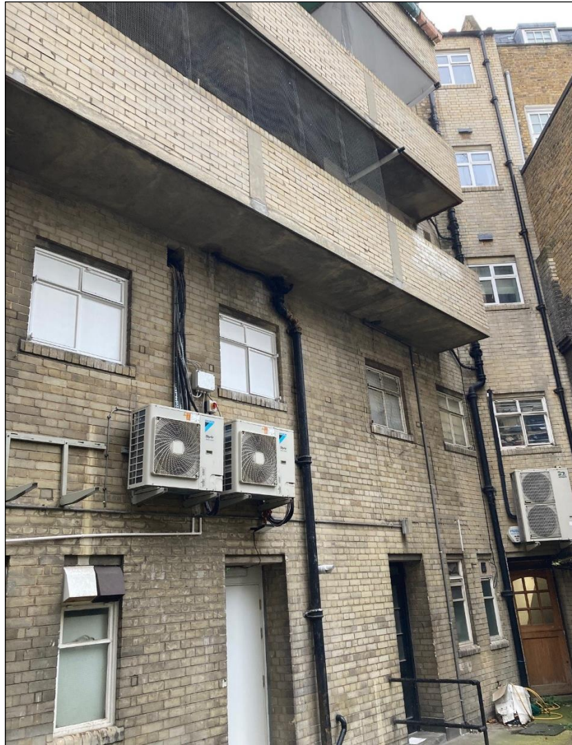
Rear view of application site showing two air conditioning units and extract fan in window.
